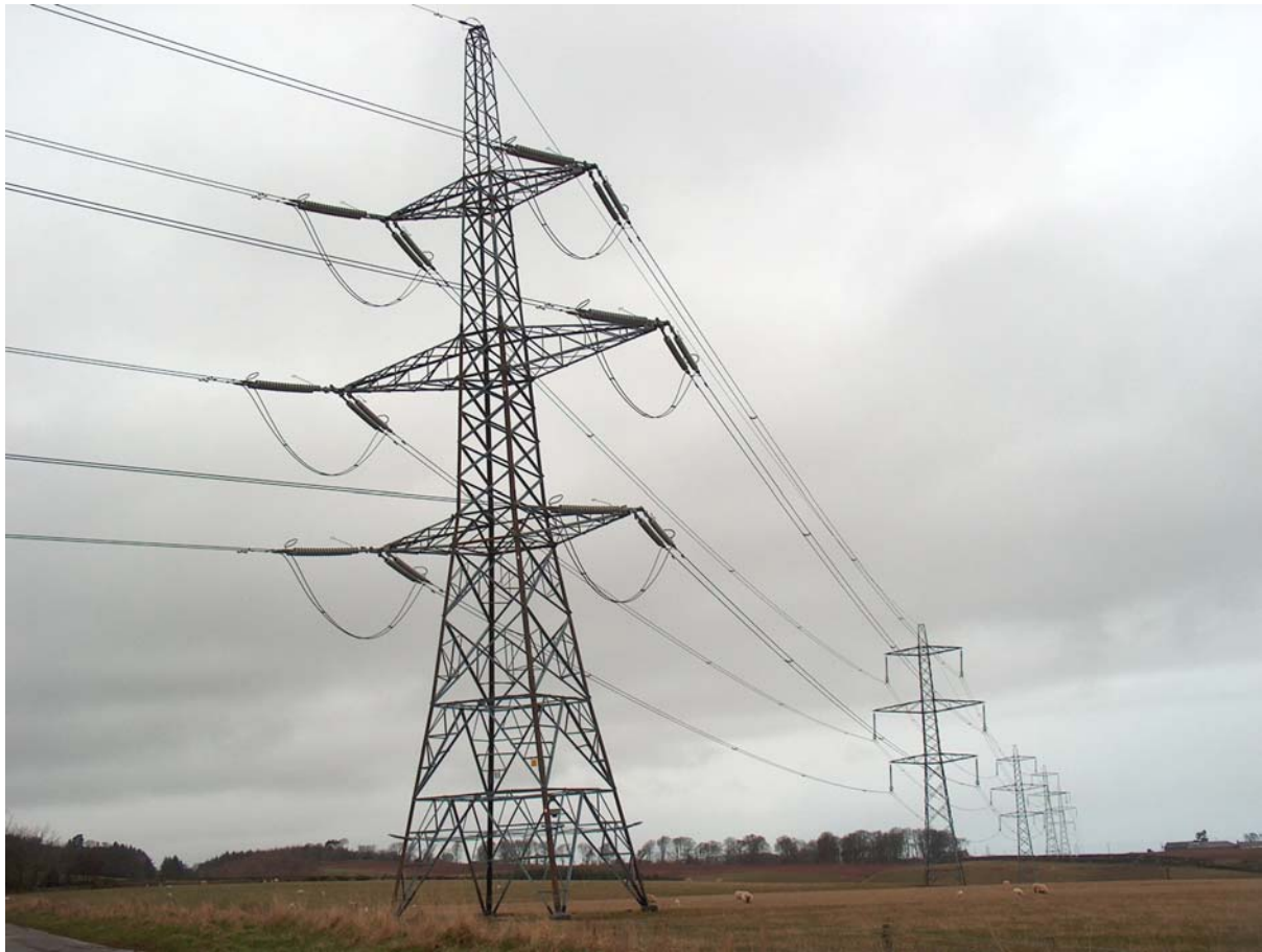
▲ Angle Tower (for change in direction) and line towers.
